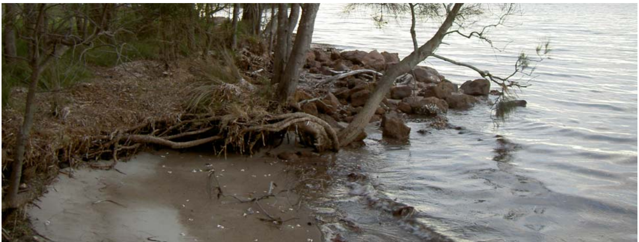
(2) Foreshore erosion around trees and dumped rock rubble.
