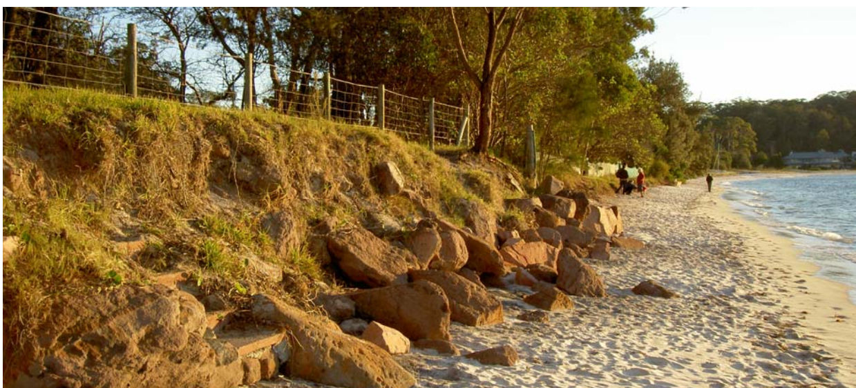
(3) Erosion of the dune and haphazard rock “protection” at the eastern end of Corlette Beach
