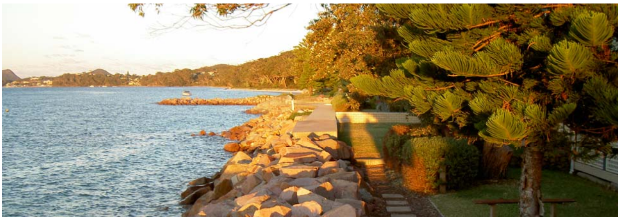
(1) Revetments and groynes protecting development on the north-eastern side of Sandy Point
