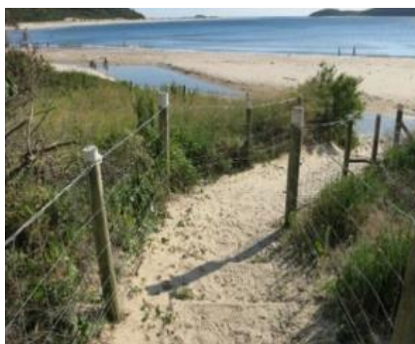
Stormwater outlet undercutting an accessway at Fingal Bay
