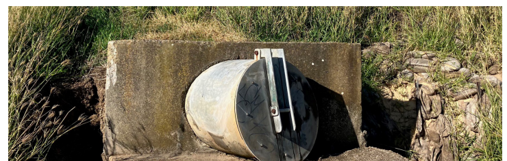
Flood gate at Raymond Terrace
