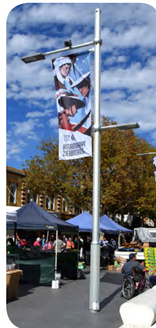
Smart Pole Lighting
