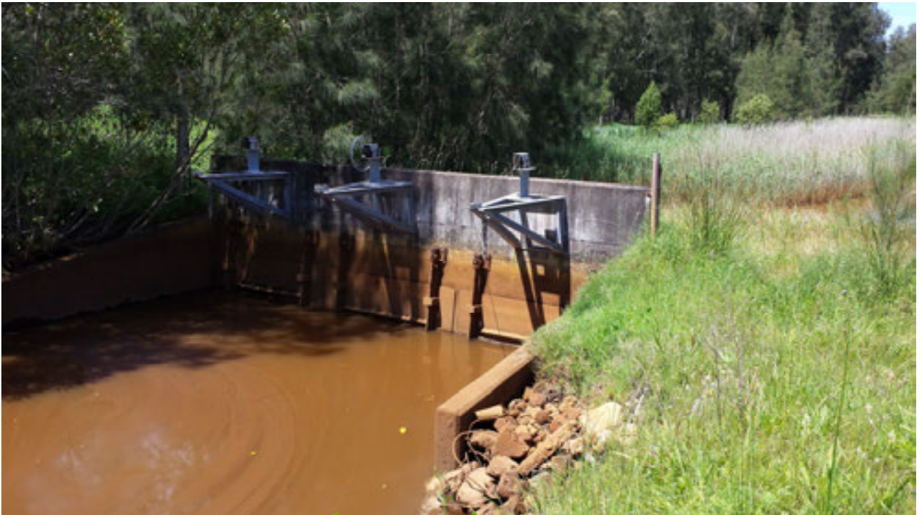
Figure 3-1 Anna Bay Main Drain floodgates
