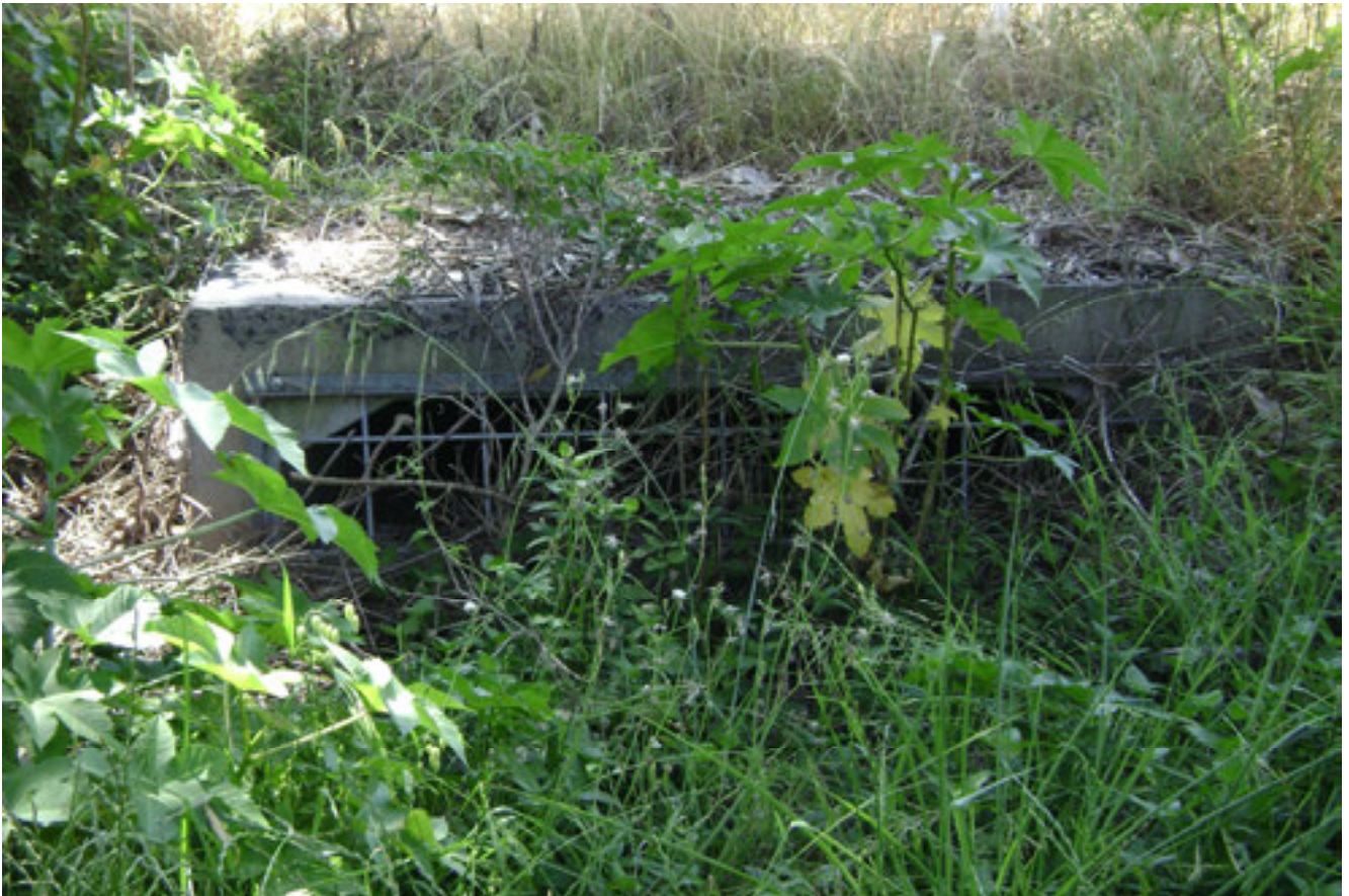
Figure 3-4 Culvert inlet portal on Fern Tree Drain in Anna Bay, partially obstructed by vegetation and debris
