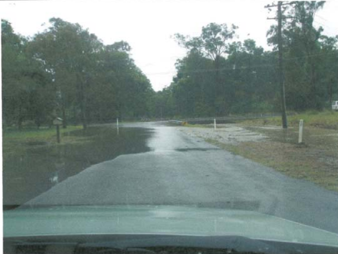
April 2008 following storm event. Water breaking out of drain in Karwin Rd flooding intersection at corner of Karwin and Kula
