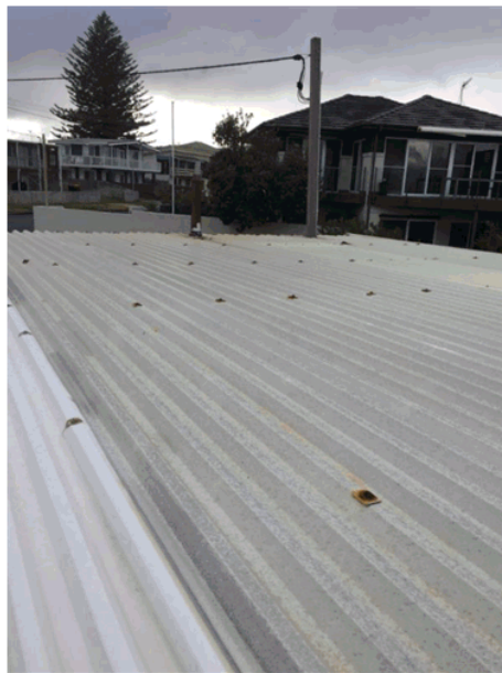
Figure 7 – Corroded roofing screws. Failing roof battens beneath sheeting.
