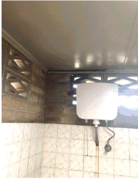
Figure 1 – Asbestos roof lining through out current building
